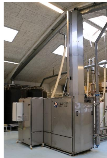
SuperOx® at Aquarden facilities in Denmark.
