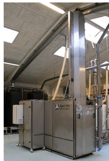
SuperOx® at Aquarden facilities in Denmark.
